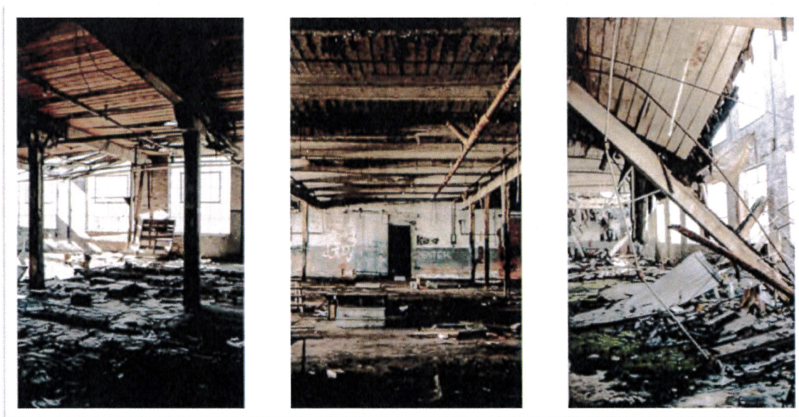
Figure 4 | Mill Conditions Prior to Recent Stabilization Efforts
